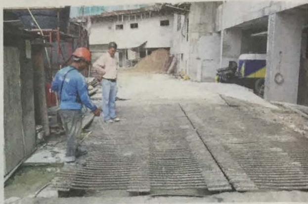
The silt traps at the construction site along Jalan Kuchai Maju 13. — Photos: LOW BOON TAT/The Star
