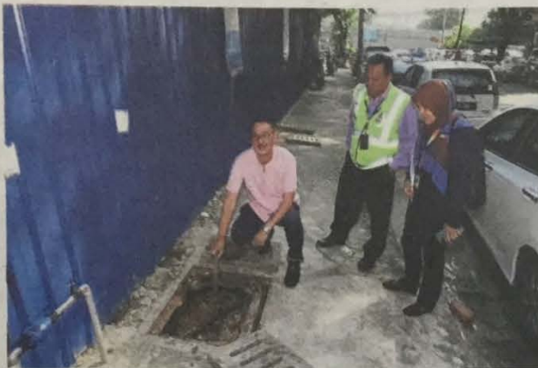
Chin showing the stagnant mass of solidified oil under the sump cover of the blocked drain in Jalan Kuchai Maju 15.
