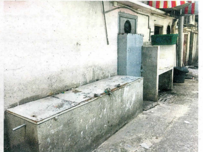
Illegal extensions along drains make it very difficult for waste contractors to do their job.
