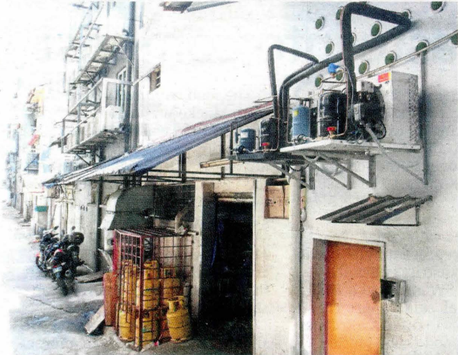
Illegal structures include grilled up cages for gas tanks and a mounted stand for the air-conditioning compressor.
