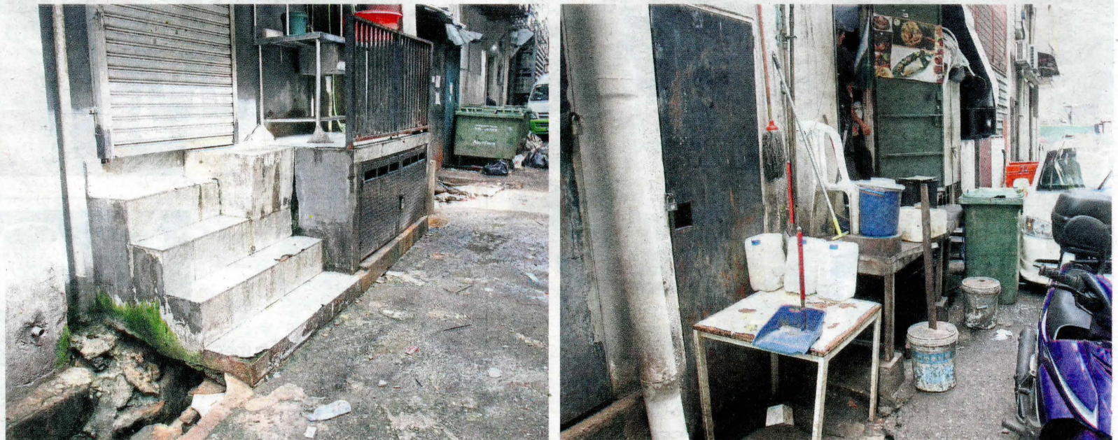
Concrete steps (left) at a back alley are blocking the drain, while (right) multiple obstacles have been identified at this premises.
