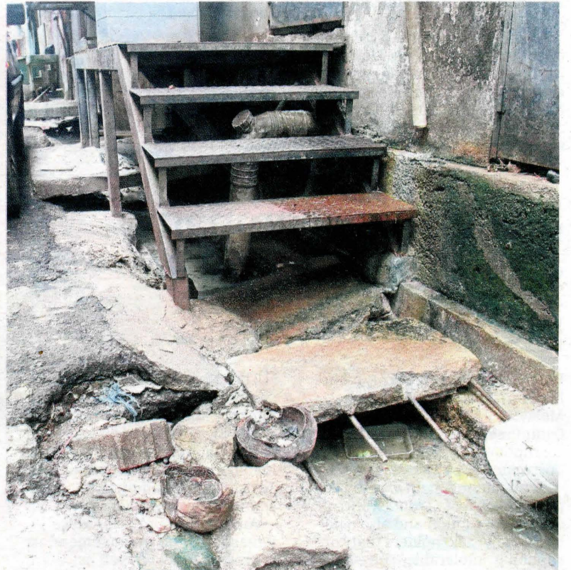
Drains here are blocked and clogged with oil and grease.
