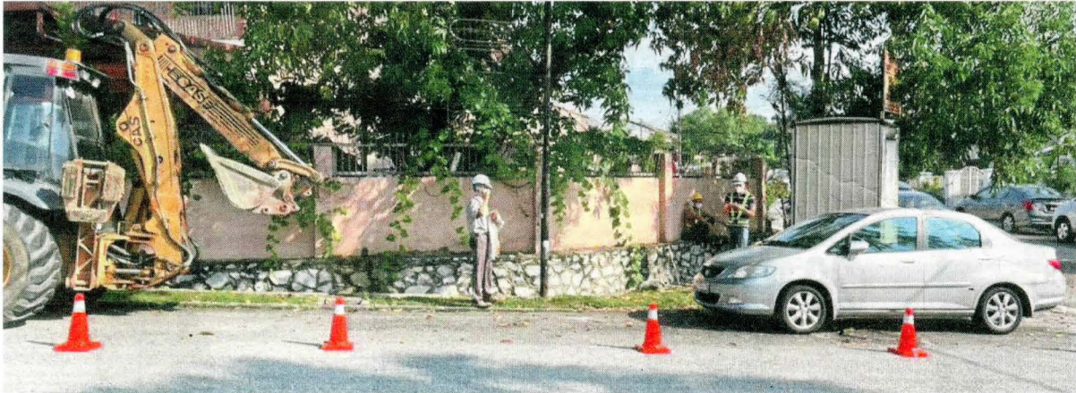
Taman Bukit Indah residents parked their cars where a pole was to be placed, to prevent its installation.
