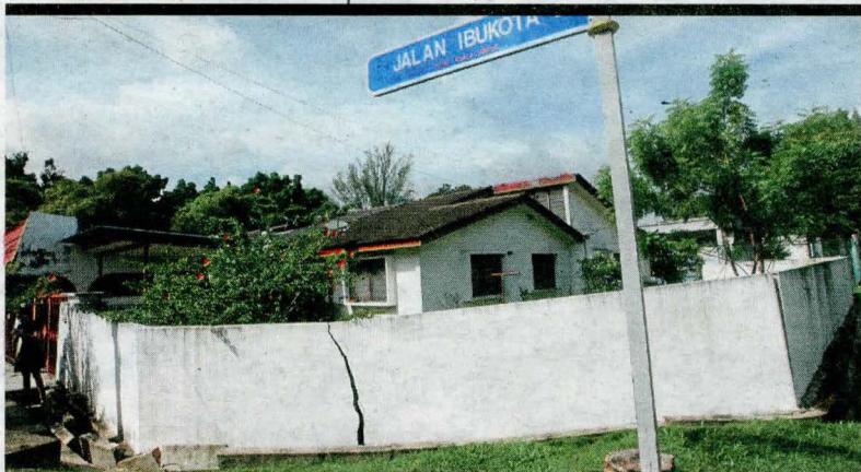
The large crack on the fence of Ng's rented house in Danau Kota, Wangsa Maju.
