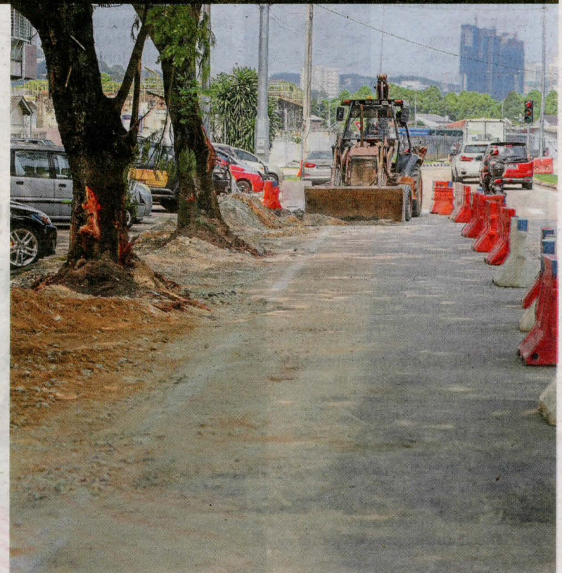
Jalan 1/40 in the process of being upgraded and beautified to create more parking space for the convenience of residents of Taman Pusat Kepong apartments. — Photos: GLENN GUAN/The Star
