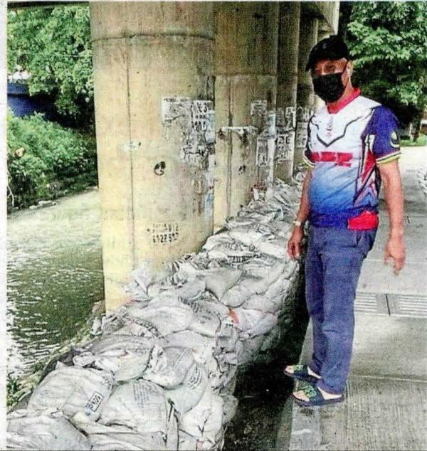
Mahadi checking on damaged sand bags in Pintasan Segambut and Jalan Rahmat, which were replaced promptly on the same day, on Sunday during his daily checks on such sites in the capital city. — Photo courtesy of DBKL
