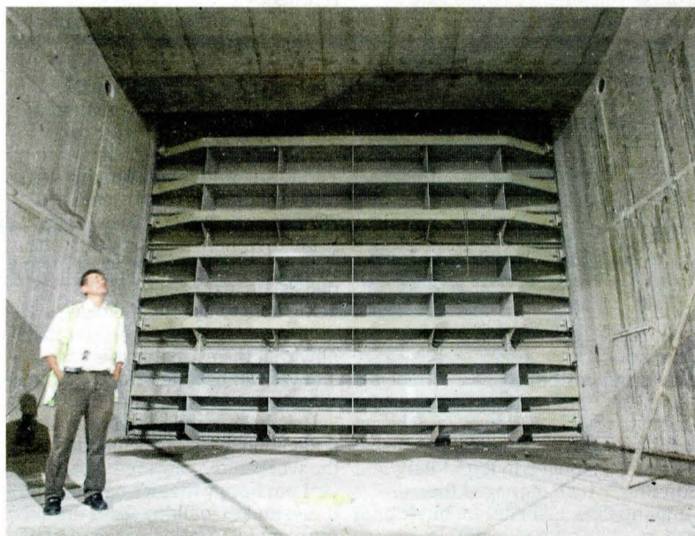
A file photo of the SMART Tunnel showing a flood gate that channels water to the Taman Desa holding pond.
