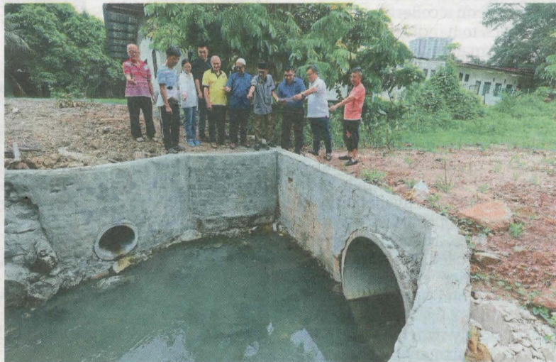
Lai (third from right), Lau (second from right) and Nasaruddin (fourth from right) checking the concrete water sump with residents of both villages. — SAMUEL ONG/The Star
