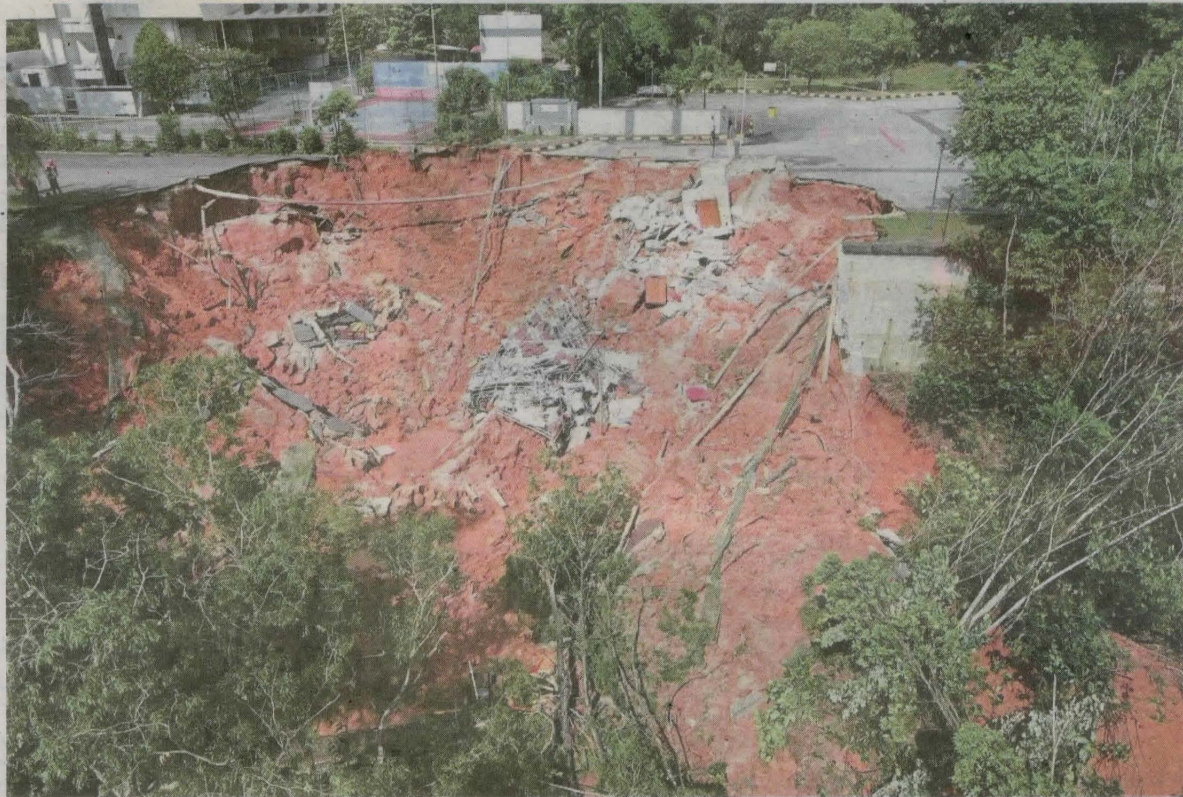
A view of the area around Persiaran Tunku Syed Sirajuddin in Kuala Lumpur, after the landslide. – Photo courtesy of the Fire and Rescue Department.
