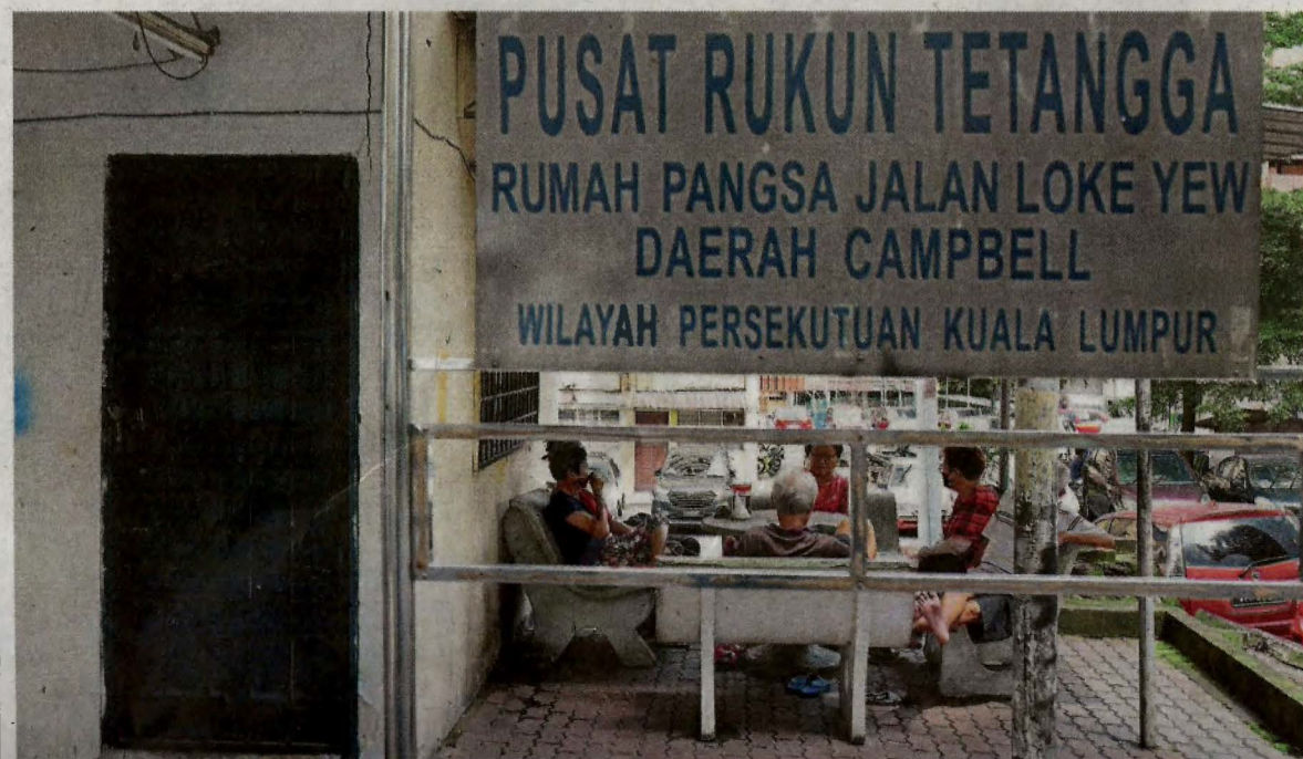
The decades-old Jalan Loke Yew flats are showing their age, say residents.
