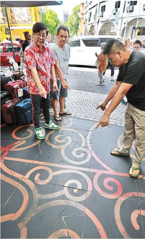
Ang (in red shirt) showing cracked tiles in Petaling Street alongside association treasurer Chan Pooi Chee (second from left) and a trader. (Right) Ang pointing out a stall's tattered cover.
