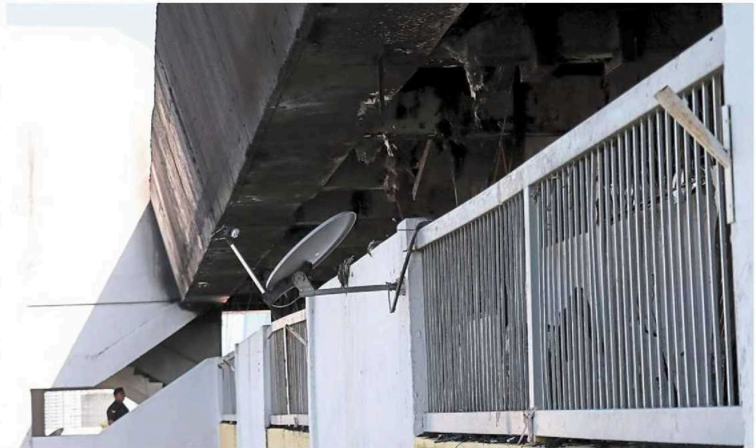
The aftermath: Initial findings found that the cause of the fire at Block 70 of the Sri Sabah flats in Cheras was not firecrackers but wiring issues, says Muhammad Salleh. — WILLIAM GARY/The Star
