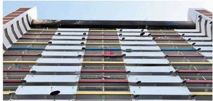
Six units of Block 70 at the 17th floor of PA Seri Sabah were destroyed in a fire. — Photos: LOW LAY PHON and WILLIAM GARY/The Star
