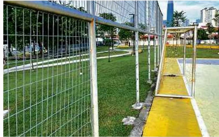
The fencing adjacent to the futsal court has been removed in an act of vandalism, presumably with the intention to sell as scrap metal. PIC COURTESY OF WRITER
