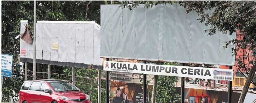
Residents want old billboards in the city removed as they pose a danger. Similar billboards are seen here in Jalah Megah Mendung, off Jalan Kelang Lama.
