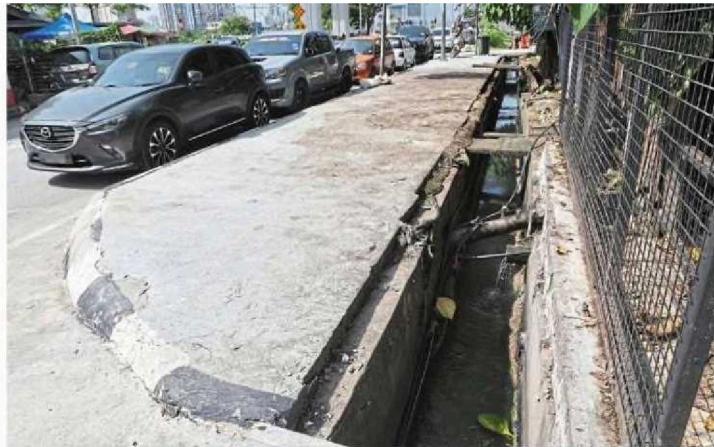
Dirty and narrow drainage along the industrial and commercial areas blamed for floods.
