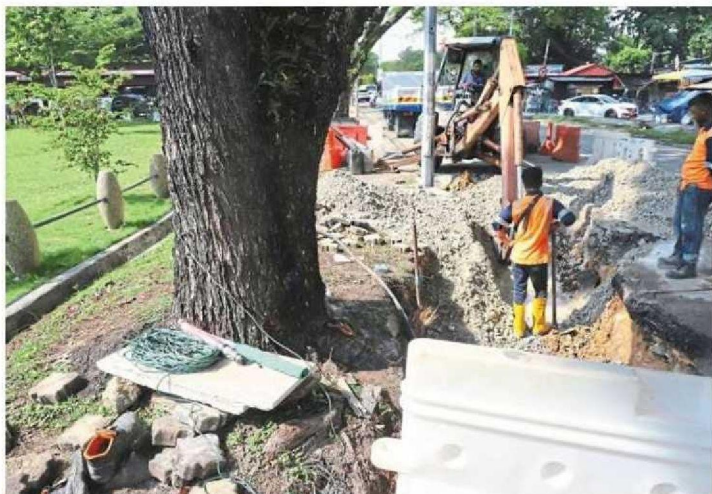
There have been incidents where repair works by utility companies have damaged old trees along Jalan Terengganu in Penang.
