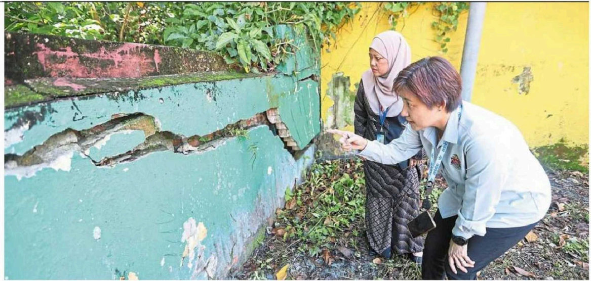
Leong with DBKL Tun Razak city branch officer Asyqah Yusuf checking the cracks on the temple wall. — LOW BOON TAT/The Star
