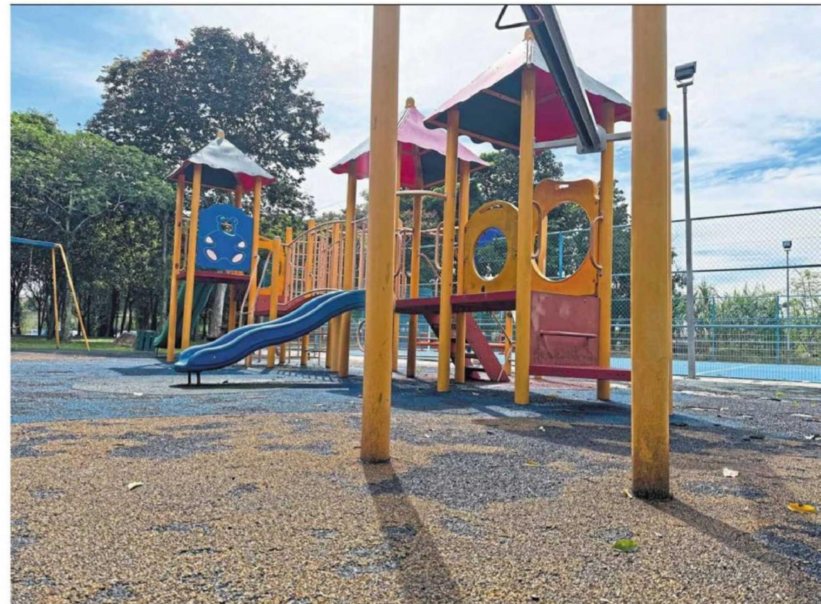
The flooring tiles at Taman Sri Segambut playground are damaged. — FARID WAHAB/The Star
