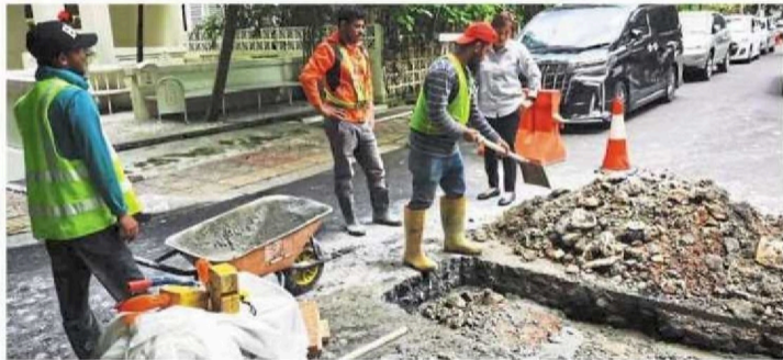
Leong (right) observing the progress of remedial roadworks in Jalan Sin Chew Kee, Kuala Lumpur.
