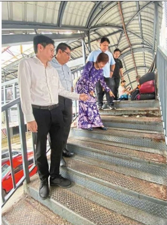
(From left) Fong, Lai and Leong checking out the pedestrian bridge in Pudu with its gaping holes and uneven flooring.
