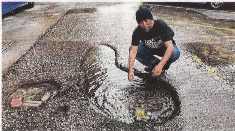
Khairul showing the pothole which has grown bigger since the underground pipe burst.
