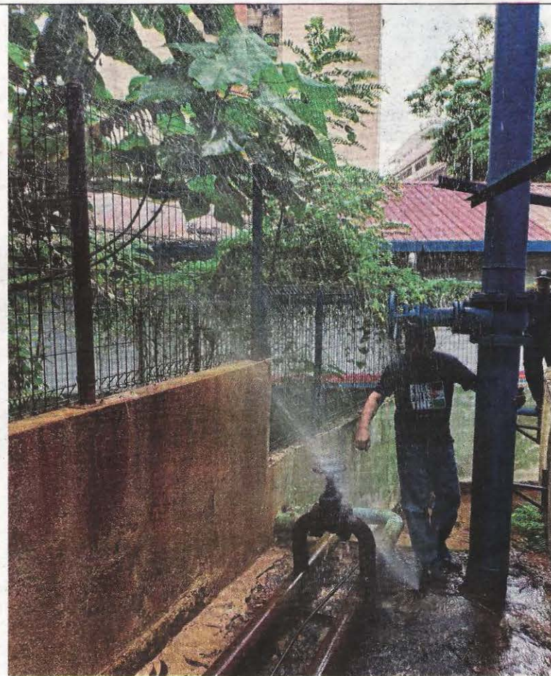
The burst pipe at the tank that supplies water to blocks A and B in Intan Baiduri PPR in Selayang.
