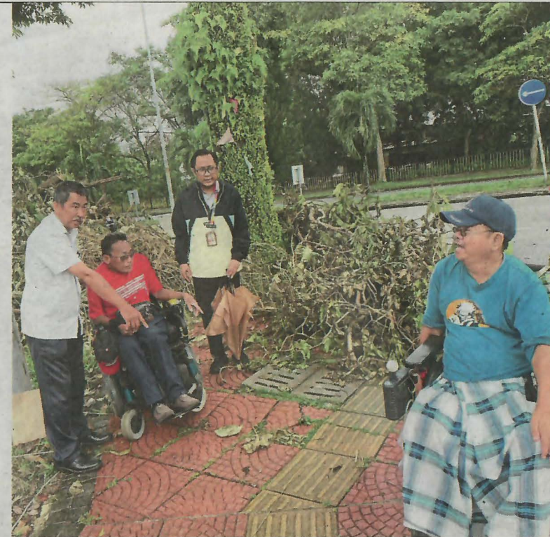
Yee (left) showing the broken and uneven tiles at the junction of Jalan Kuang Bertam and Jalan Metro Prima. With him are Mohd Nor and two wheelchair users.
