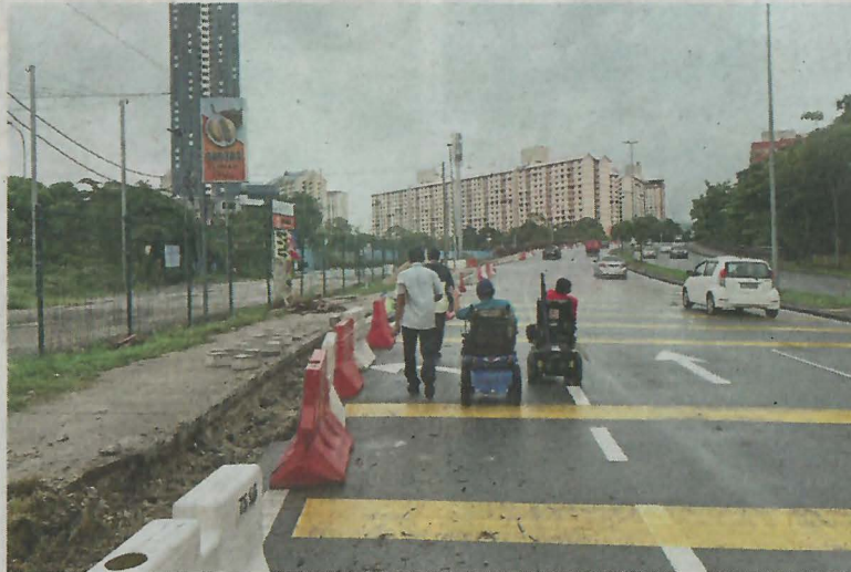
Wheelchair users unable to access the pavement have to use Jalan Metro Prima despite proximity to fast-moving traffic on the road.
