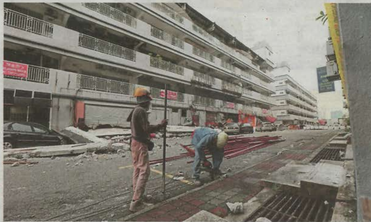
Workers setting up a temporary barrier at Block A of the Sri Desa Entrepreneurs Park. The area has been barricaded with yellow tape to prevent unauthorised entry. — Photos: YAP CHEE HONG/The Star
