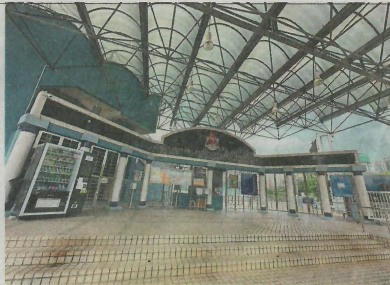
The 35-year-old complex in Bandar Tun Razak is undergoing major mechanical and electrical works.
