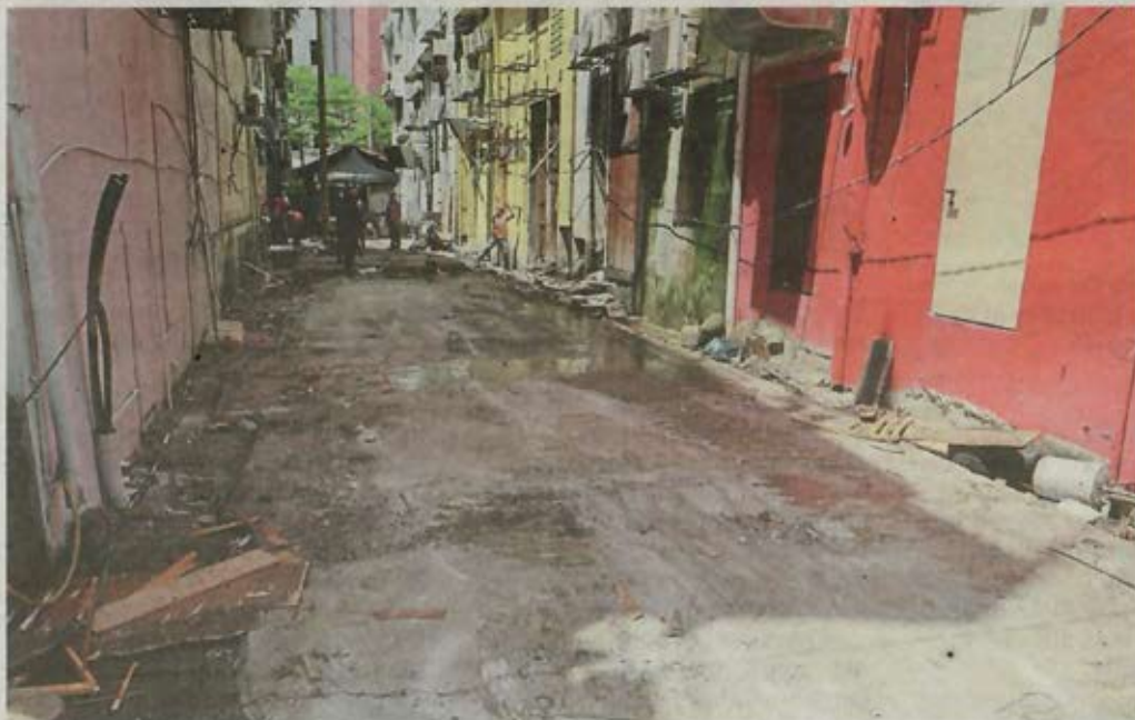
Lorong Baba now free of obstacles following the joint operation by government agencies.
