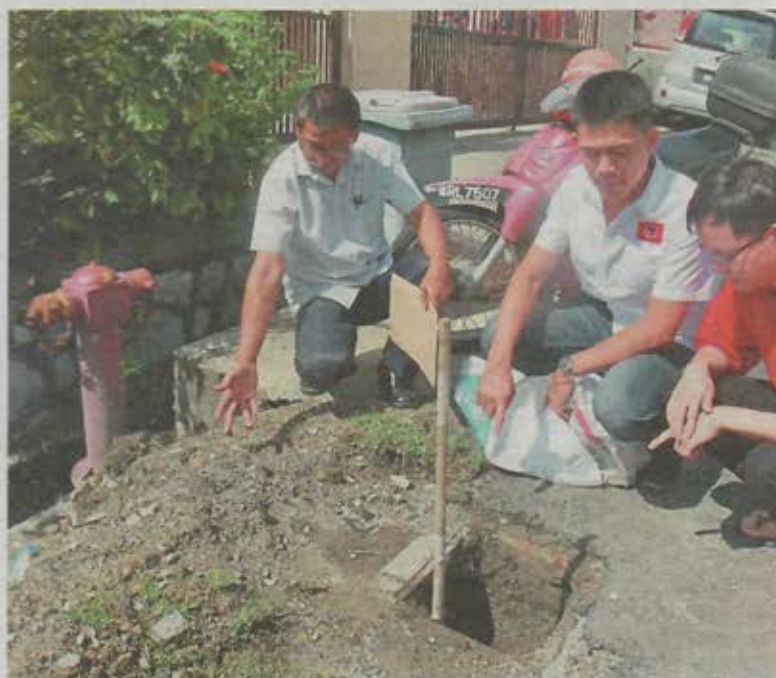
Yee (left) pointing to the faulty fire hydrant at Jalan Jinjang Permai 9. — KAMARUL ARIFFIN/The Star
