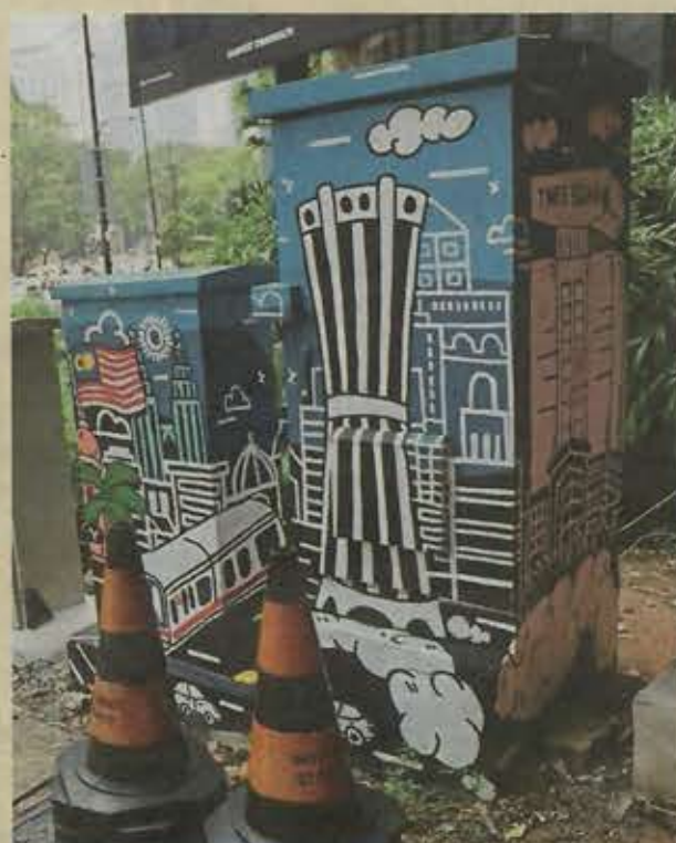
The facade of these feeder pillars and sub switchboard panels in Kuala Lumpur now sports a cheerful look.
