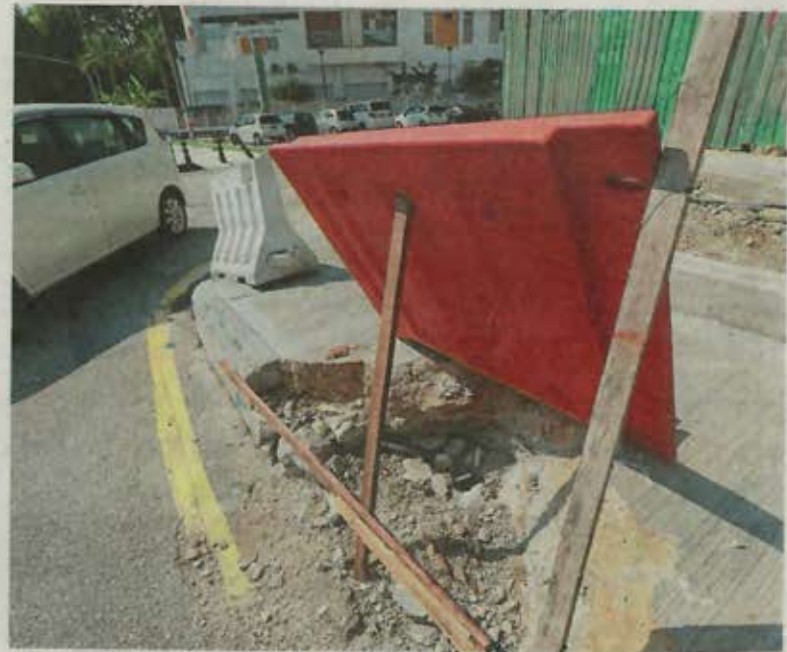
Many scupper drains in Jalan Maarof meant for flood mitigation were blocked with cement. It is now being removed after stakeholders complained to DBKL.
