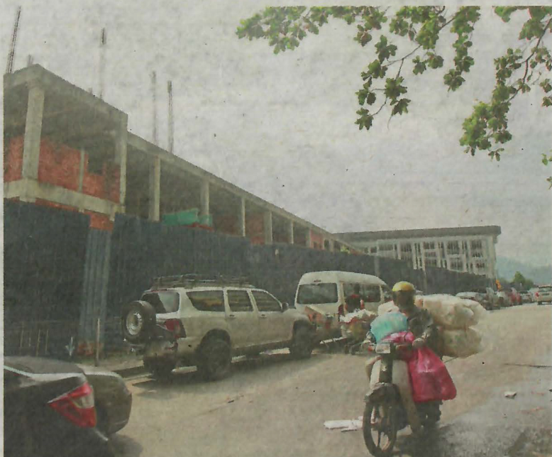
The integrated halal abattoir project site is surrounded by hoarding, with little to no construction activity going on.
