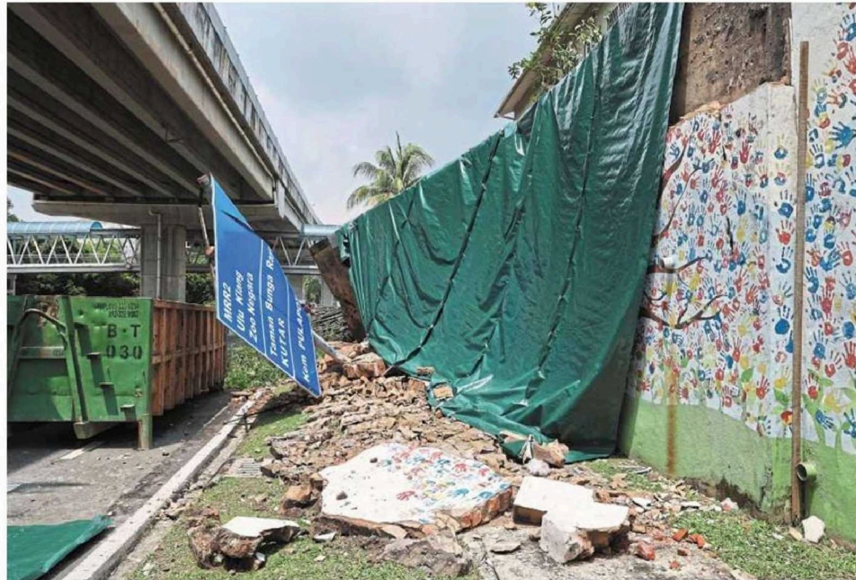
The collapsed slope along Jalan Genting Klang damaged the retaining wall, which featured a patriotic mural, and a number of street signs. — ART CHEN/The Star
