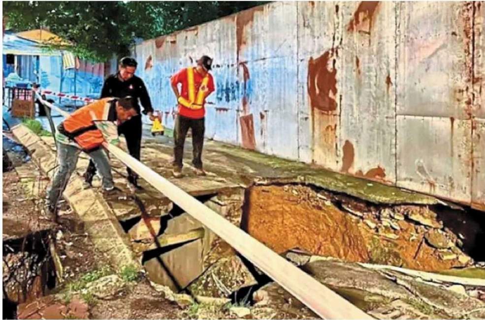
Unsafe pavement: Workers inspecting the collapsed drain in Jalan Pantai Permai.
