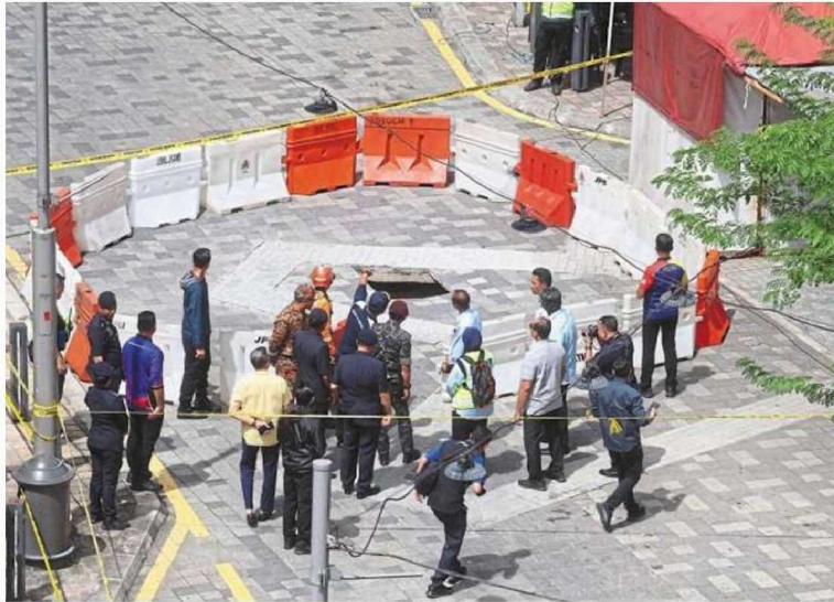
Another danger zone: The sinkhole found about 50m away from the first incident. — LOW BOON TAT/The Star
