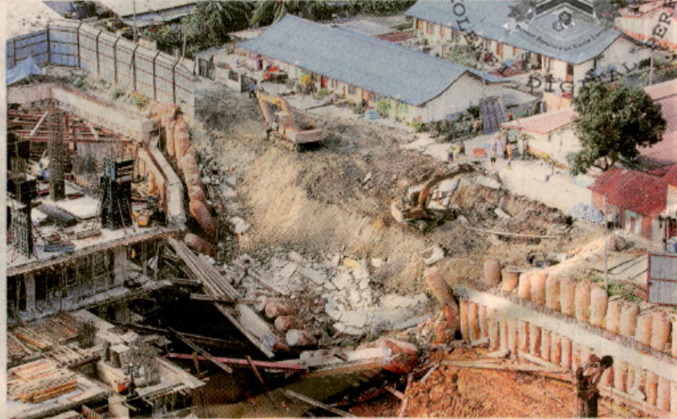
The developer will submit a report on the cave-in, which will be studied by an independent consultant appointed by City Hall.
