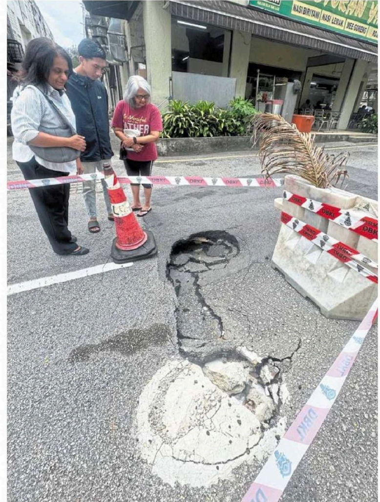
(From left) Pereira, Quwais and Netto at the sinkhole on Jalan 6/132 in Gasing Indah, Kuala Lumpur.
