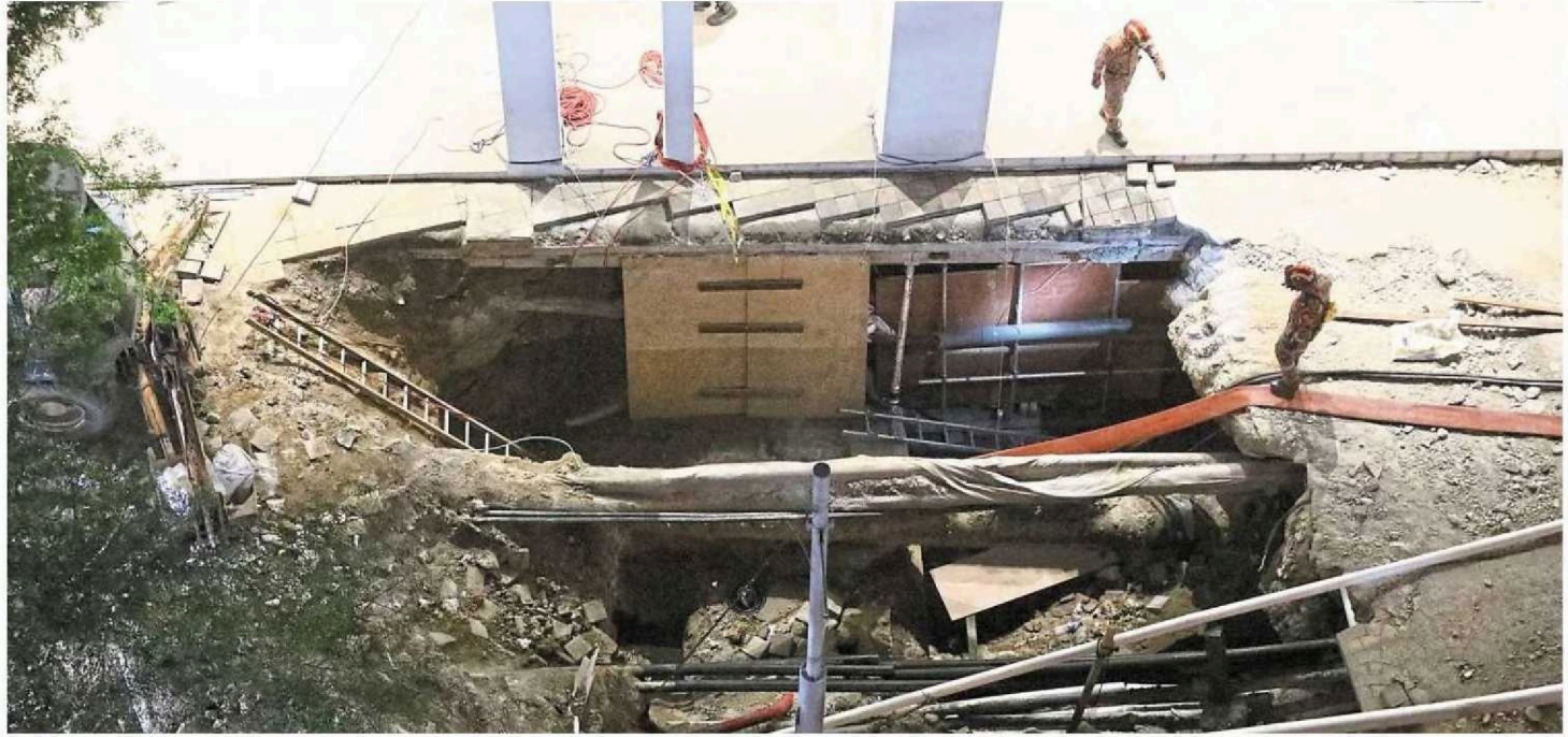
The RM10mil allocation under Budget 2025 for a geotechnical study of soil structures in Kuala Lumpur's Golden Triangle follows a recent spate of land subsidence and landslides, including the tragic case of a woman who fell into a sinkhole in Jalan Masjid India in August. — Filepic
