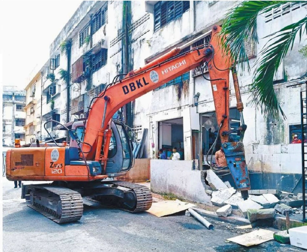
A DBKL excavator demolishing an illegal extension at Jalan Angsoka in touristic Bukit Bintang.
