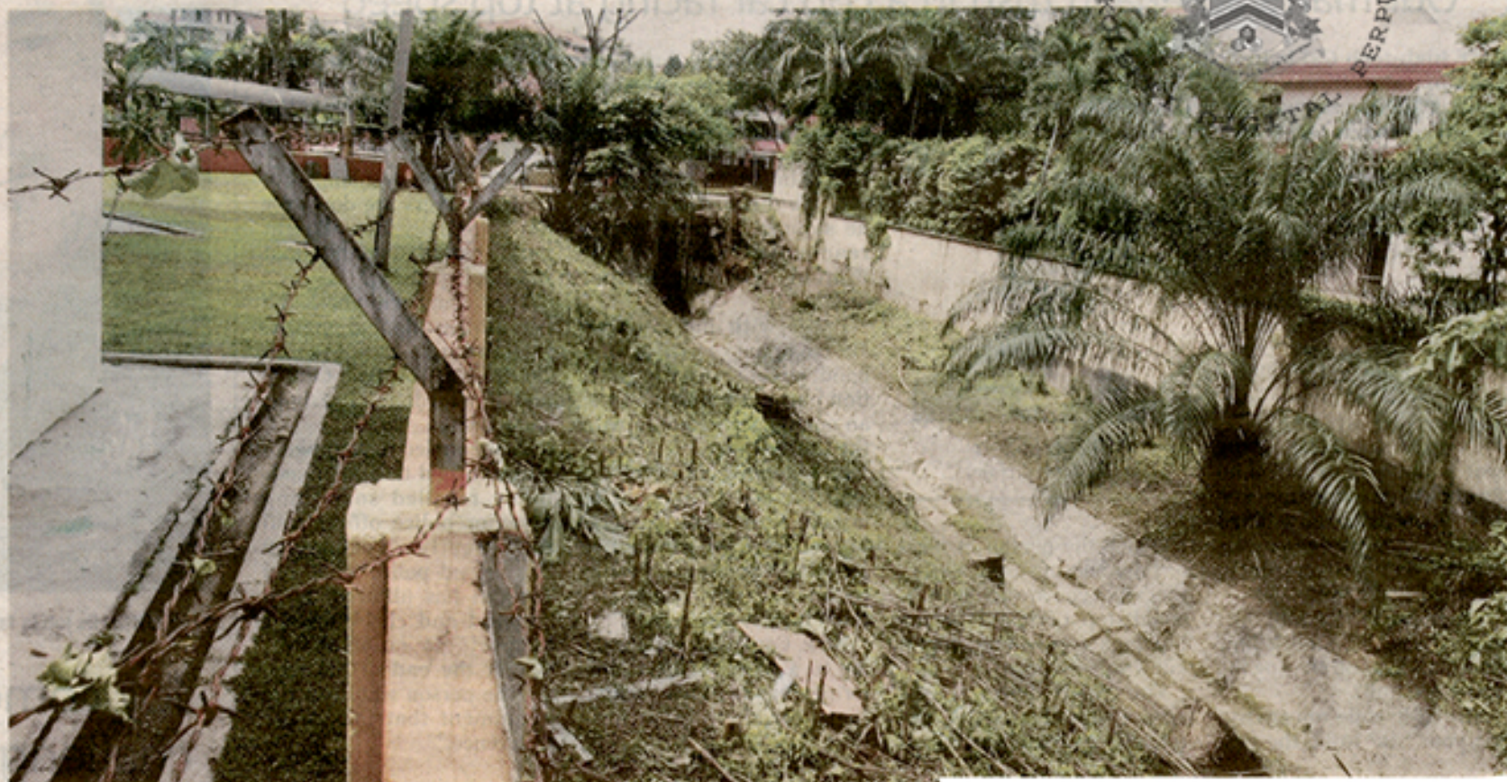
SHODDY WORK: The incomplete clean-up behind the walls of SK Bukit Damansara
