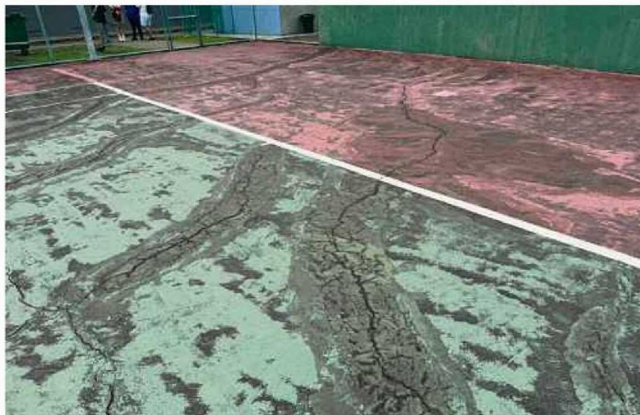
Many of the tennis courts at the Titiwangsa Sports Complex have deep cracks and are covered in slippery moss. PIC COURTESY OF KUALA LUMPUR LAWN TENNIS ASSOCIATION
