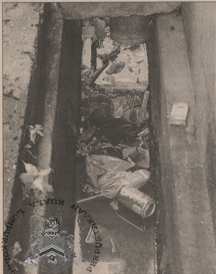
STUCK: One of the many clogged drains in the area.
