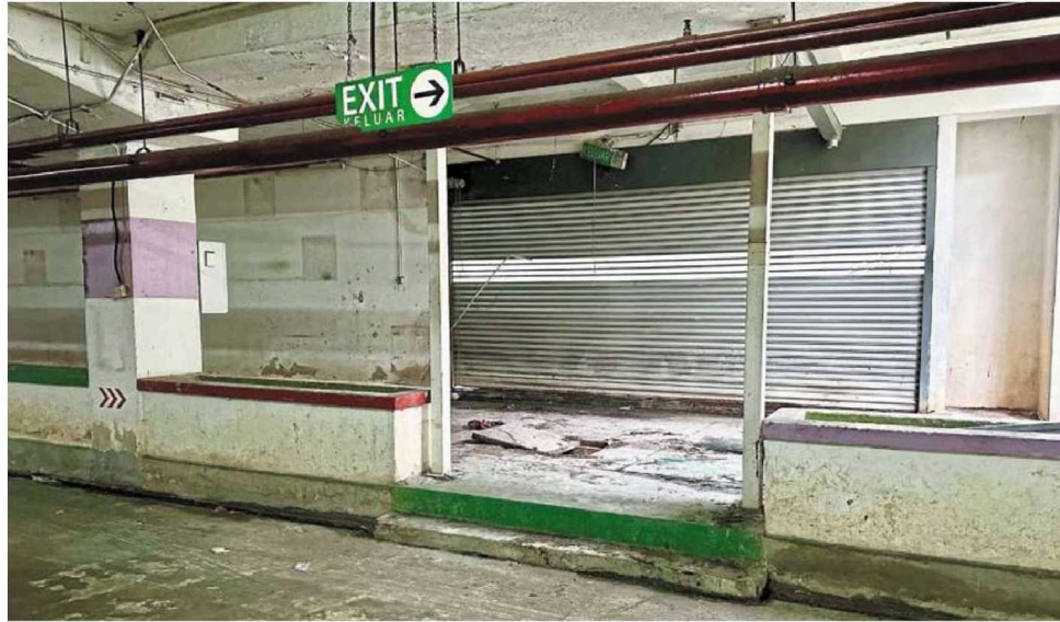
Poorly lit and dotted with cracked tiles, the underground parking facility beneath Dataran Merdeka has become a cause for concern. — Photos: SHAARI CHEMAT/The Star
