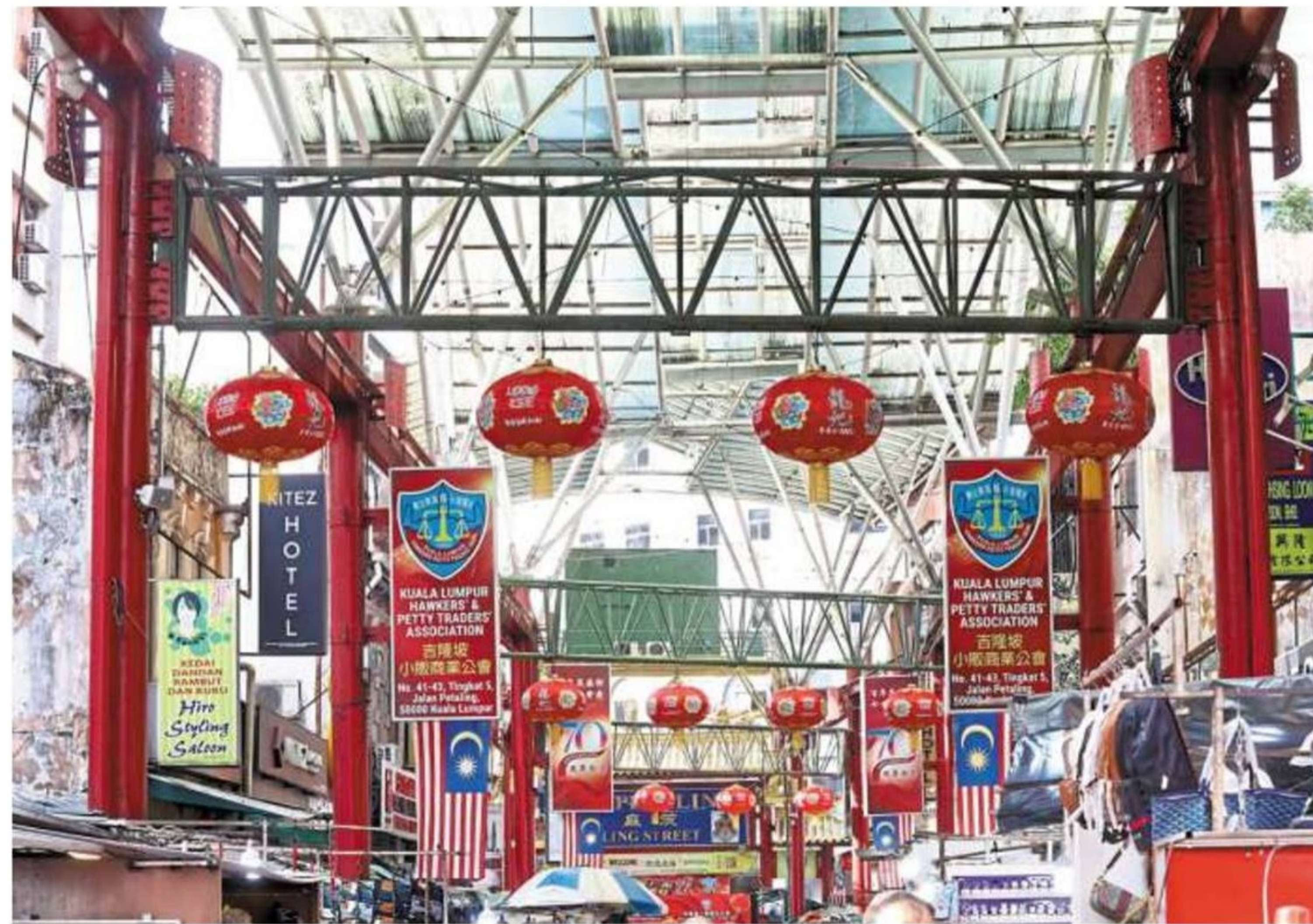
Parts of the roofing over Petaling Street are dirty or damaged. — Filepic
