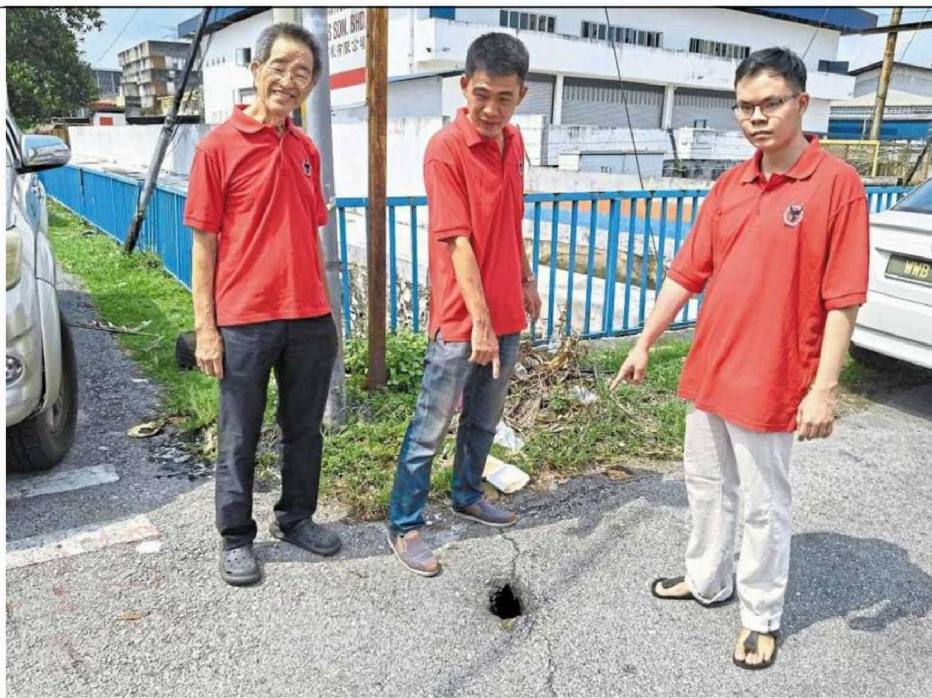
(From left) Koh, Lee and Chua standing next to the sinkhole in Jalan Jinjang Aman 5 in Kepong, Kuala Lumpur.
