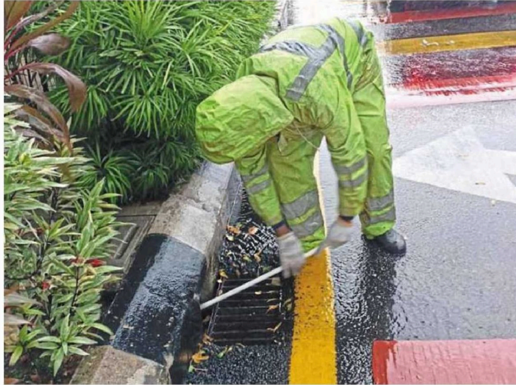
A DBKL worker clearing the drain of debris following flash floods in several areas in the city on Monday.
