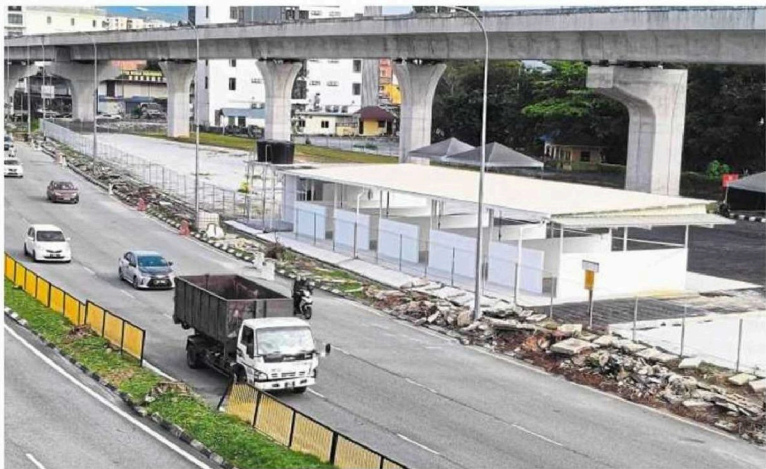
The structure was allegedly built over a gas pipeline and near Jinjang Fire and Rescue Station in Kepong, Kuala Lumpur.
