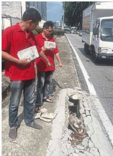
Lee (left) and Kepong PRM chairman Chua Yi Ken looking at the caved-in verge.
