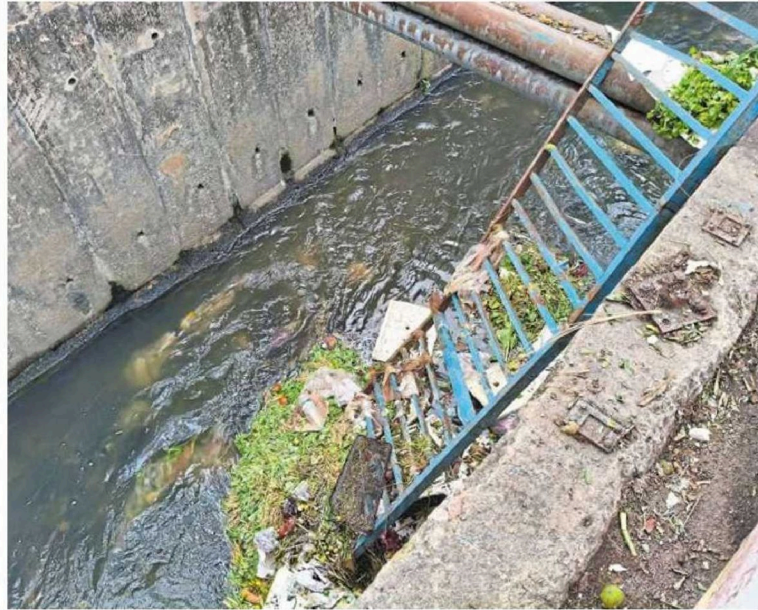
The damaged guard rails along a monsoon drain in the back lane of Jalan 2/3a in Pusat Bandar Utara Selayang, Kuala Lumpur.
