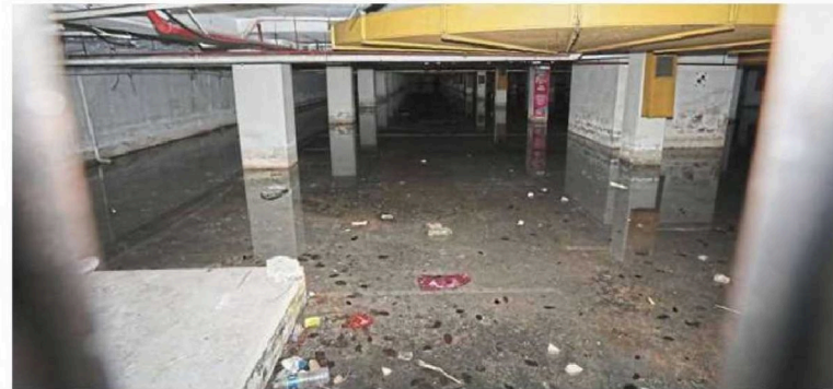
The flooded basement carpark of the old Lucky Plaza is now a breeding ground for mosquitoes and a pool filled with rubbish.
